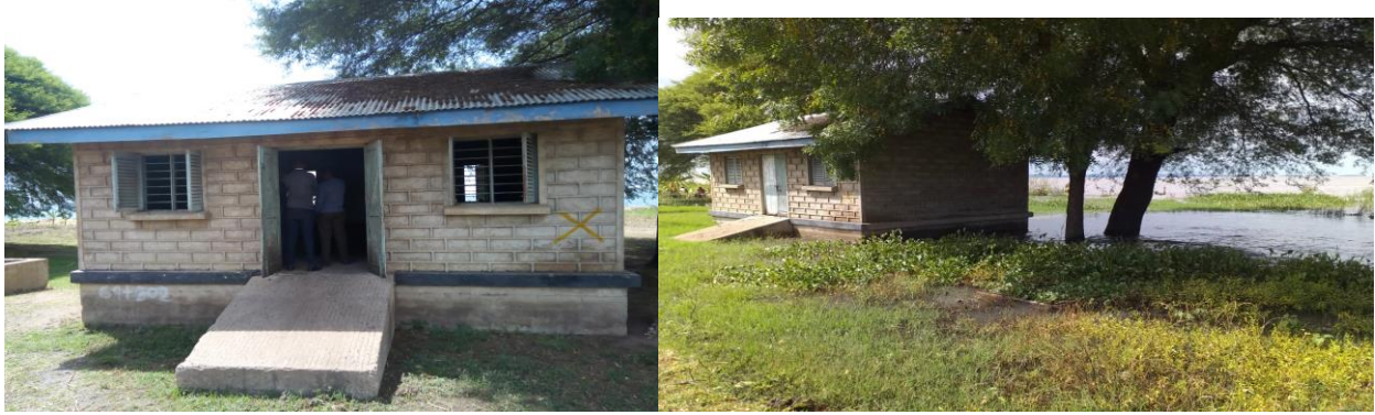
Figure 9: The observed effect the recent rise in Lake Victoria water levels to the pump houses at Kasahunga,, water sources. The sources were designed in 1970s without integration of climate change issues in during the design. The proposed intervention under output 1.1 avoids such mistake, and considers projected /future climate events under various scenarios including optimistic ones. The photo on the left-hand side was taken in July 2019 before the rise of lake water levels while the photo on the right hand was taken in February 2020 after the rise of Lake water levels due to floods and extreme precipitation events.
